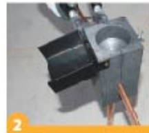
2 Insert the copper wire to inside of the thermowelding mold and put the earthing electrode to down side of the mould
